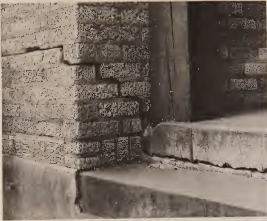
Figure 17.—Foundation cracking caused by the high shrink-swell potential of Pecos silty clay loam, nonsaline, 0 to 1 percent slopes.
