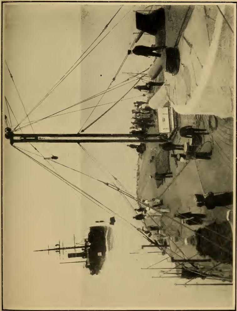
A TEMPERLEY-MILLER MARINE CABLEWAY COALING H. M. S. "TRAFALGAR" AT SEA A carrier, from which are slung the sacks of coal, is hauled backwards and forwards by steel ropes stretching between the foremast of the transport and a mast rigged on the warship.
