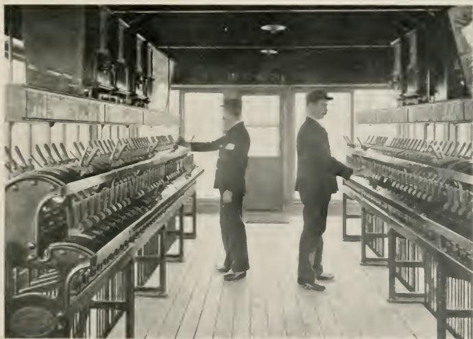
INTERIOR OF AN ELECTRIC SIGNAL-CABIN, L. AND N. W. R.
