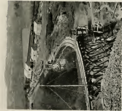
THE TEMPORARY ROAD, BEING USUALLY LAID WITH AS MUCH SPEED AS POSSIBLE, AFFORDS VERY ROUGH TRAVELLING.
