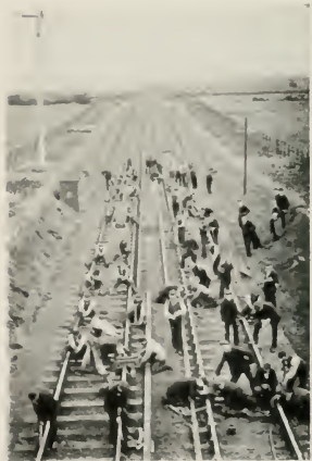
PREPARING THE PERMANENT WAY FOR ELECTRIC TRACTION NEAR NEW- CASTLE, NORTH-EASTERN RAILWAY.
