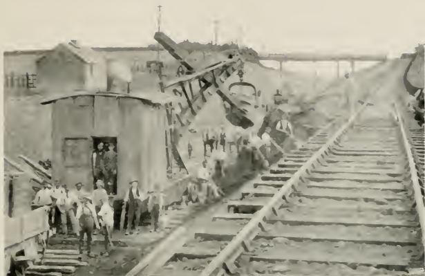
THE EXCAVATION OF A NEW LINE OF RAILWAY IS COMMENCED AND PROCEEDED WITH IN SUCH A WAY THAT A TEMPORARY LINE CAN BE LAID DOWN AS EARLY AS POSSIBLE. ON NEARLY ALL JOBS IT IS CUSTOMARY TO BRING A "STEAM NAVVY" ON TO THE WORKS.
