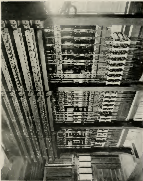
INTERIOR OF "ALL-ELECTRIC" INTERLOCKING FRAME ("CRAWLEY" SYSTEM), L. AND N. W. R.
