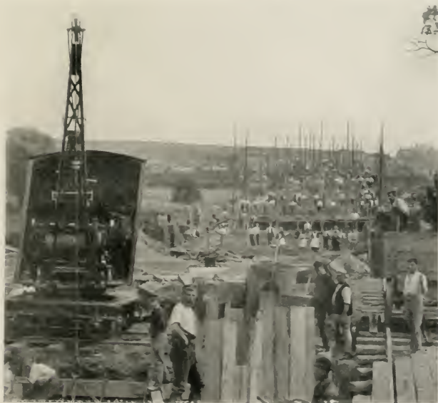
WHERE A VIADUCT HAS TO BE BUILT, THE WORK IS PUSHED FORWARD
