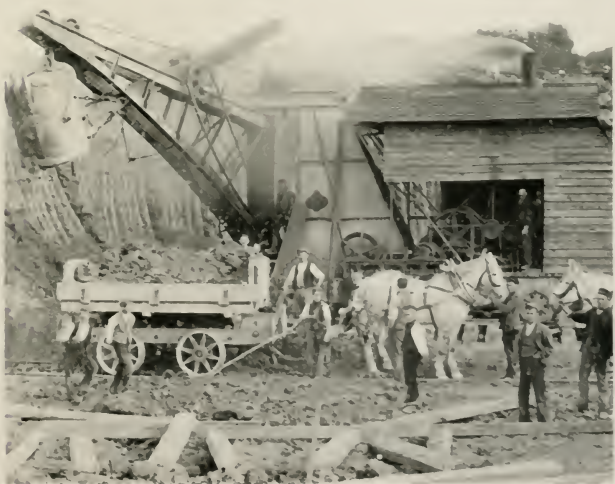
AT THE COMMENCEMENT, HORSES PULLING "TIP-WAGONS" ARE WORKED BETWEEN THE FACE OF THE EXCAVATION AND THE "TIP-HEAD" WHERE AN EMBANKMENT IS BEING FORMED.
