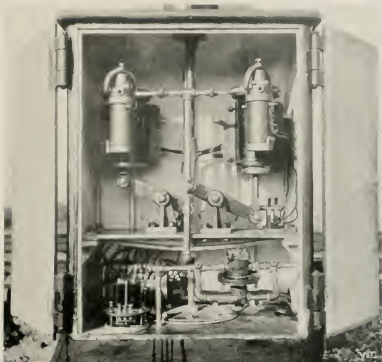
AUTOMATIC SIGNALS. VIEW SHOWING WORKS INSIDE BASE OF SIGNAL, L. AND S. W. R.
