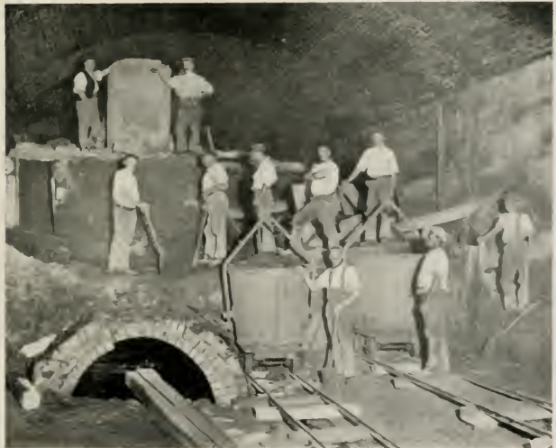
WITH "CUT AND COVER" THE WORK IS DONE FROM THE TOP. FINALLY THE REMAINING EARTH, VULGARLY CALLED THE 'DUMPLING,' IS REMOVED.
