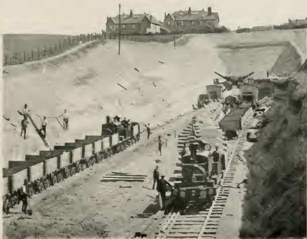
LATER ON, LOCOMOTIVES ARE BROUGHT UPON THE SCENE, WHERE THE "MUCK" (EXCAVATED MATERIAL) HAS TO BE HAULED FOR SEVERAL MILES. THE TRAIN OF EMPTIES IS TAKEN BACK TO THE CUTTING, AND A THIRD TRAIN, WHICH HAS BEEN FILLED IN THE MEANTIME, IS THEN READY TO BE DESPATCHED.
