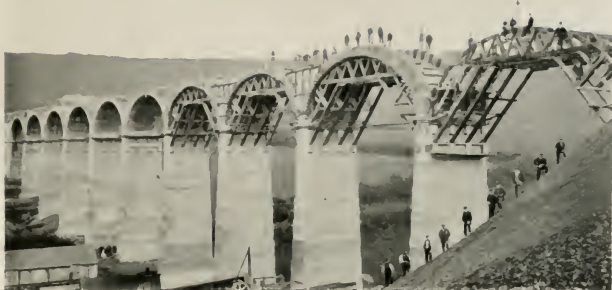
THE ERECTION OF A CABLEWAY IS OCCASIONALLY ADOPTED TO FACILITATE THE CONSTRUCTION OF A VIADUCT.
