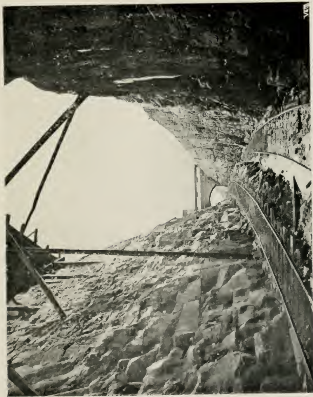
IF MUCH ROCK HAS TO BE REMOVED, BLASTING IS USUALLY THE METHOD EMPLOYED FOR DISLODGING IT.
