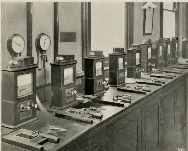
THE ELECTRO-PNEUMATIC TUBE SYSTEM FOR THE COLLECTION AND DELIVERY OF RAILWAY TELEGRAMS. THE INSTRUMENTS INSTALLED BY MESSRS. REID BROTHERS AT PADDINGTON, LONDON, G. W. R.
