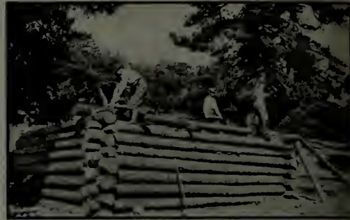
Putting up the walls. The trees used were straight young pines about forty feet in height
