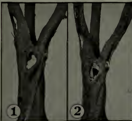
No. 1. This tree had started to decay. The owner saw this, but did not realize that it required scientific treatment. So he allowed an untrained man to "patch the holes" with cement. This "patching" was worse than useless—it was positively harmful.
