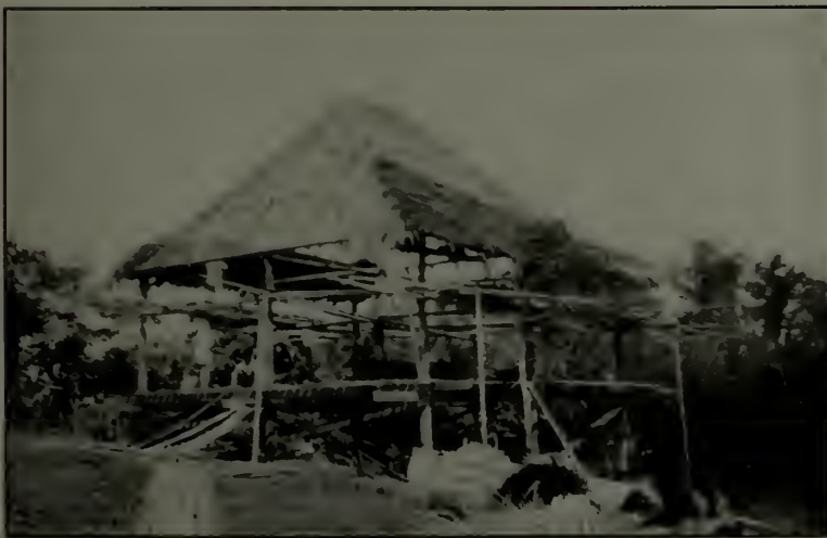
The split bamboo foundation of the roof, upon which the nipa shingles are tied
