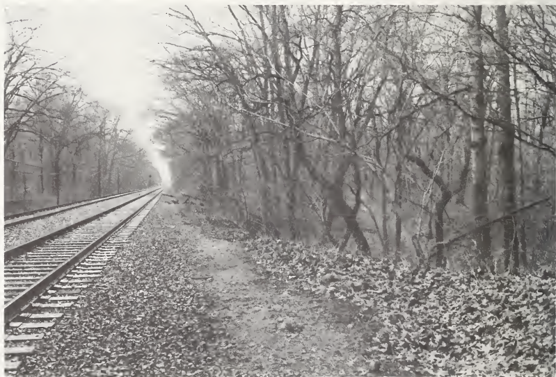
2. RR ROW - Encroaching Vegetation - Looking East
