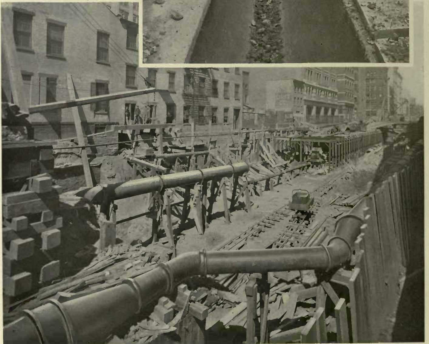
LARGE GAS AND WATER PIPES, RELAID BEHIND EACH SIDE WALL ON ELM STREET
