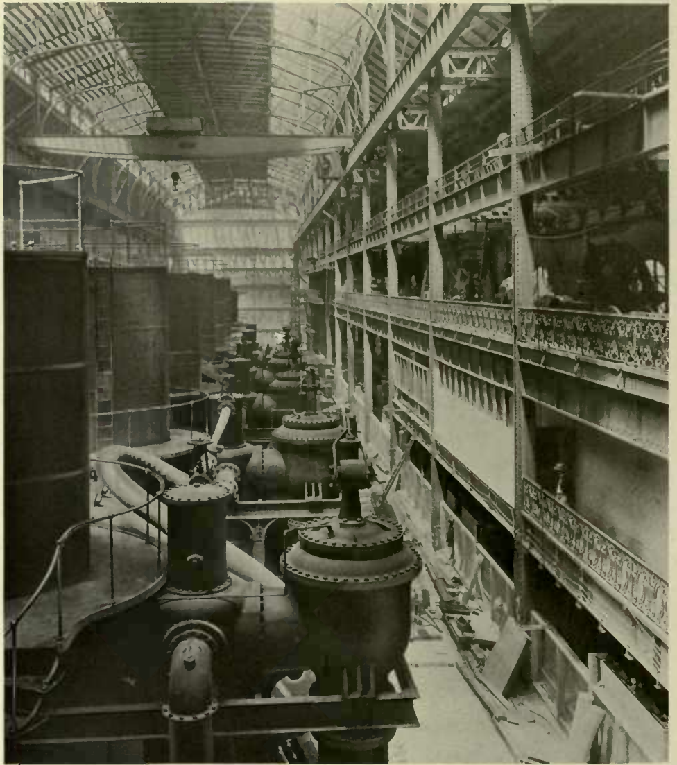
OPERATING ROOM SHOWING CONDENSERS — POWER HOUSE
