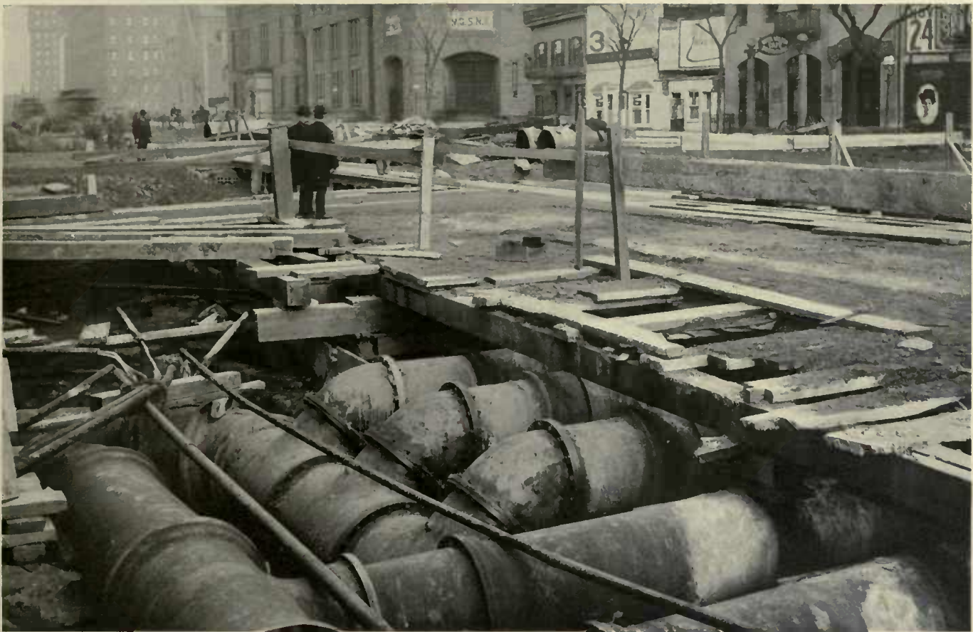
SUBDIVISION OF 36" AND 30" GAS MAINS OVER ROOF OF SUBWAY—66TH STREET AND BROADWAY
