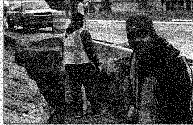
Marcus Irving, a worker at Highway and Safety Services, Inc., was unemployed before being hired to help build stormwater control systems for Montgomery County.
