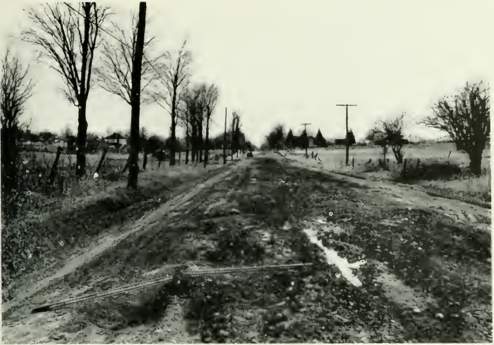
Typical broken section of roadbed caused by spring break-up conditions.
