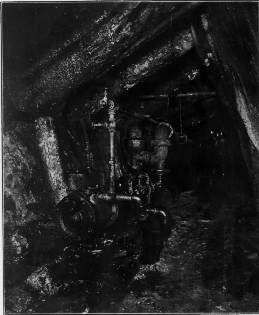
HORIZONTAL PLUNGER STATION PUMP, 250-FT. LEVEL
