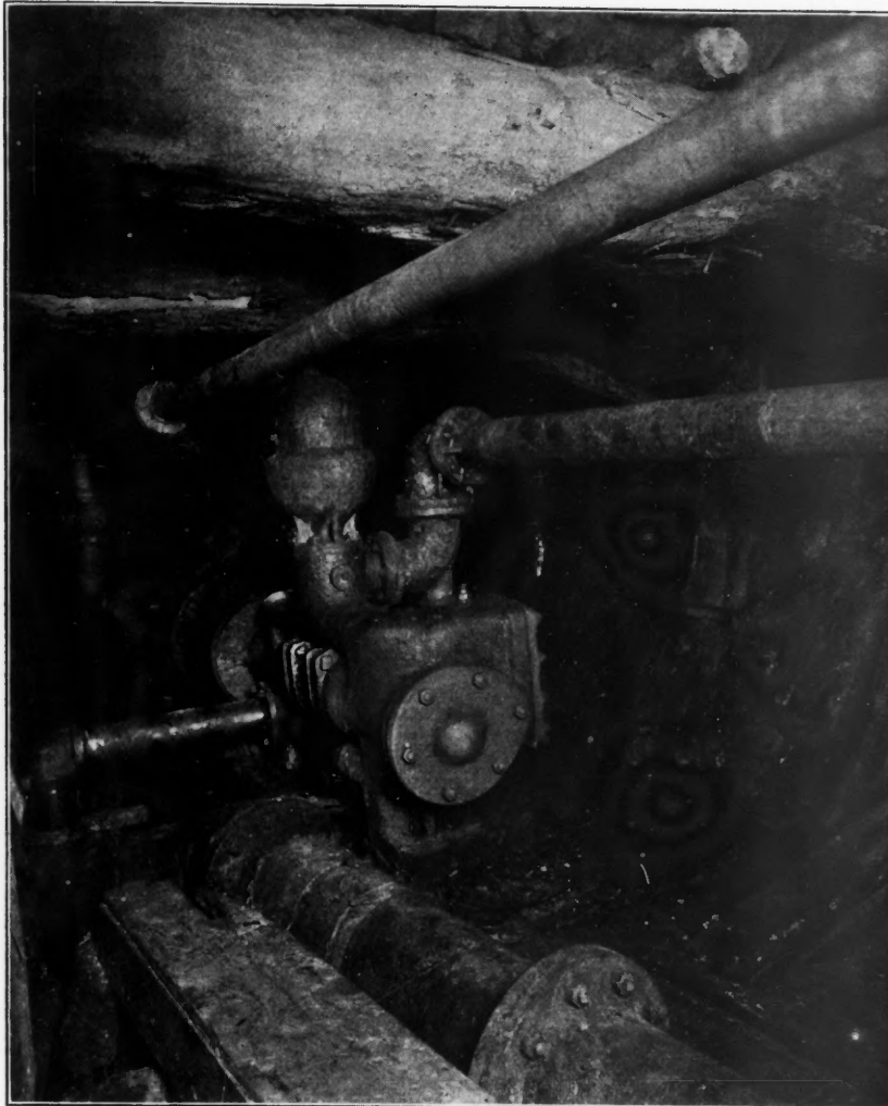
CAMERON PUMP ON THE 600-FT. LEVEL
