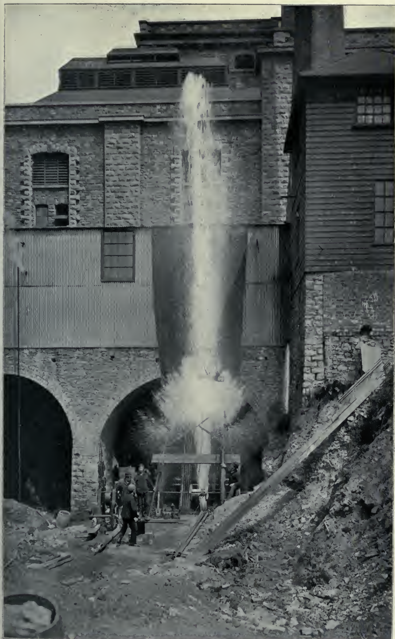
EXPLODING A CARTRIDGE IN A DEEP BORING TO INCREASE THE YIELD OF WATER.
