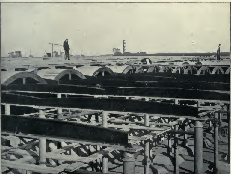
THE IRON COLUMNS AND GIRDERS THAT SUPPORT THE ROOF, WITH THE CENTERING TO FORM THE ARCHES.
