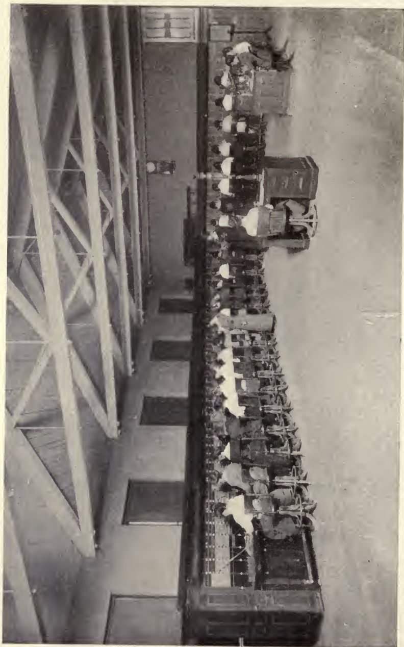
FIG. 55.—MULTIPLE SWITCHBOARD (Stromberg-Carlson)
