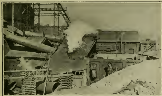
STACK BLOWN DOWN AND ROOF WRECKED BY HIGH WINDS.
