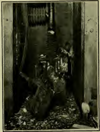
BREAKDOWN OF A HIGH VOLTAGE POTENTIAL TRANSFORMER.
