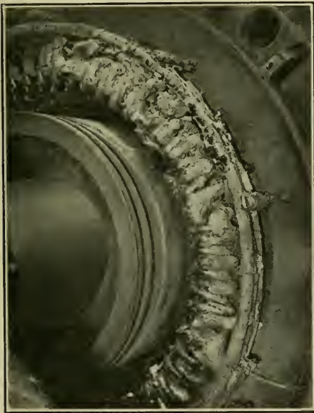
FAILURE OF LARGE TURBO-GENERATOR.
