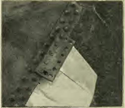
SOFT PATCH USED IN AN UNSUCCESSFUL ATTEMPT TO REPAIR A LONGITUDINAL SEAM CRACK.
