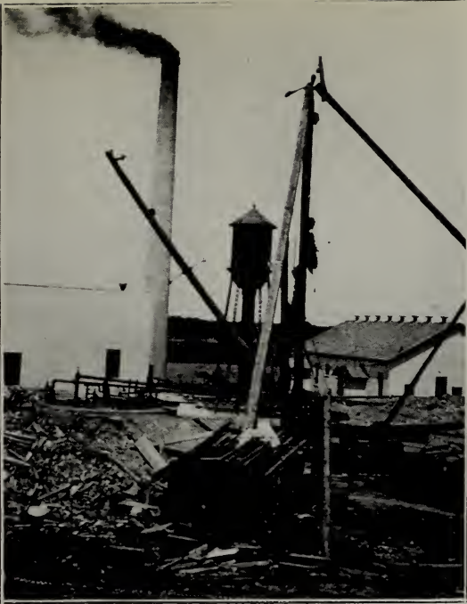
A. SINKING A CONCRETE SHAFT AT THE CROFT MINE, NEAR CROSBY PHOTO BY CARL ZAPFFE
