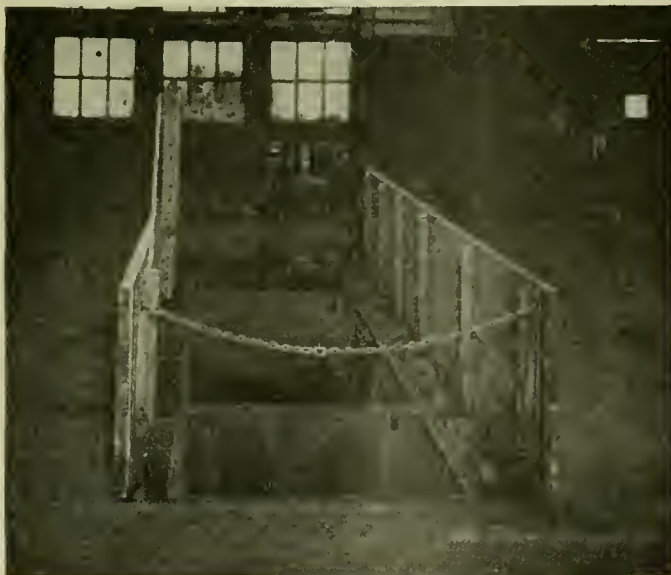
Fig. 3—Underground Type Tube Cleaner with Covers Raised
