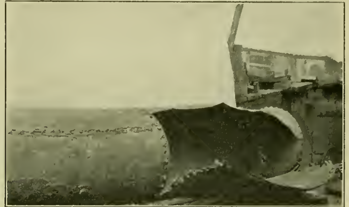
Corroded Main Air Reservoir Which Exploded, Causing the Death of One Person
