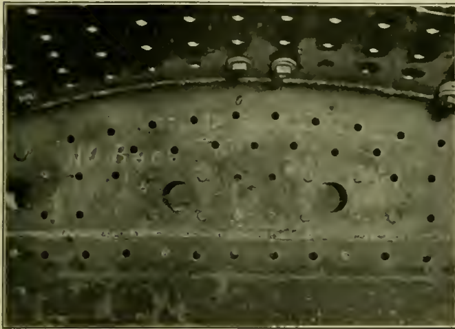
Fig. 3—Example of Direct Overhead Welding at Junction of Crown Sheet and Fire Door Sheet in Locomotive Firebox
