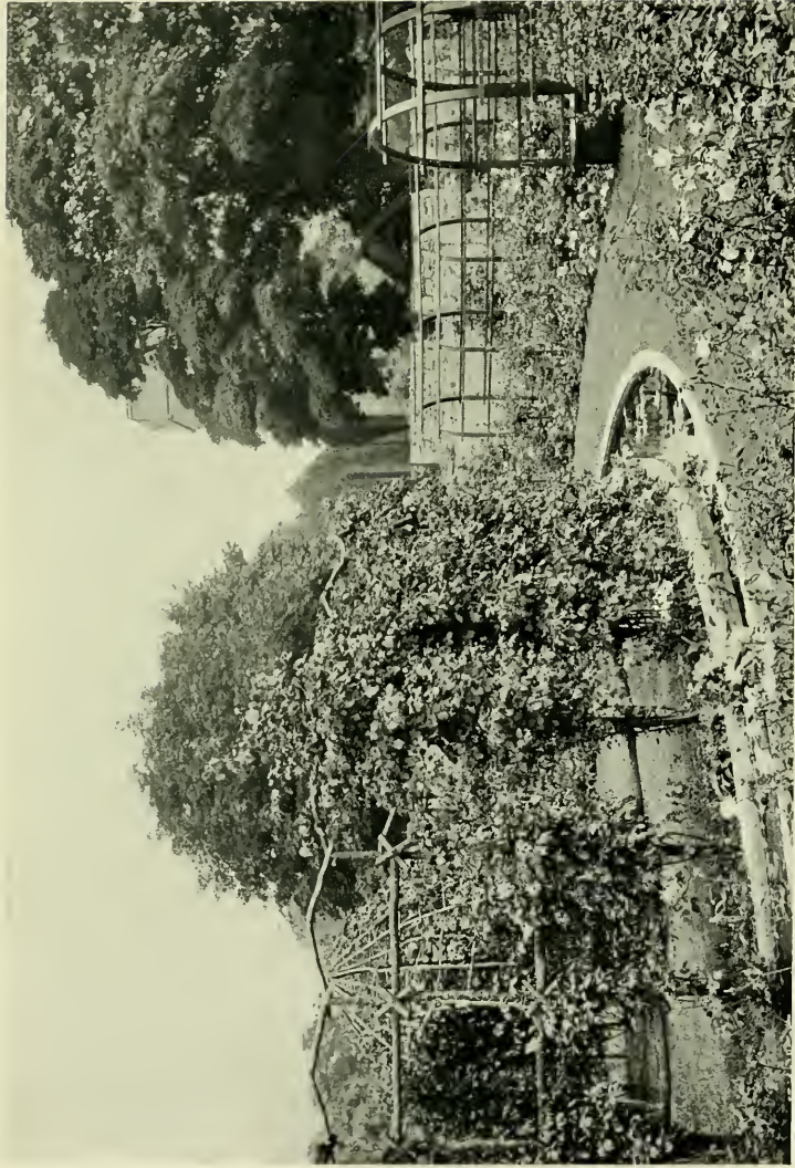
A ROSE GARDEN IN THE MAKING; SHOWING FRAMEWORK OF POLES AND LATHS.
