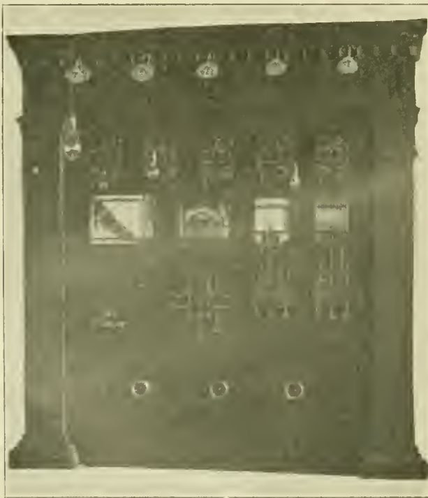
NEW BRICK SWITCHBOARD.
