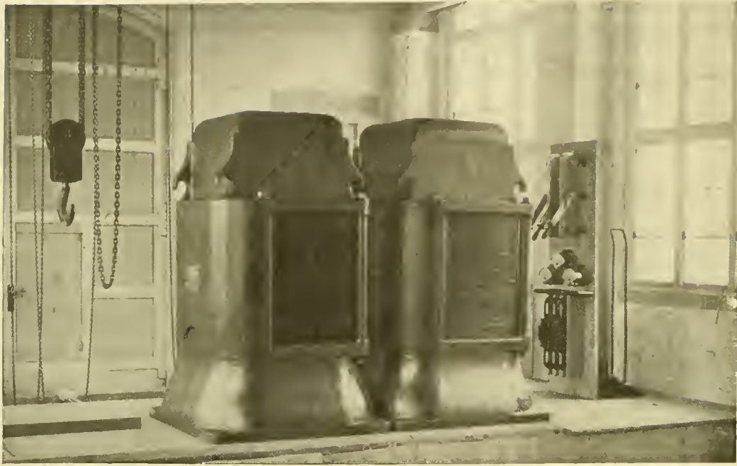
FIGURE 1—STEP UP TRANSFORMERS AT NIAGARA.
