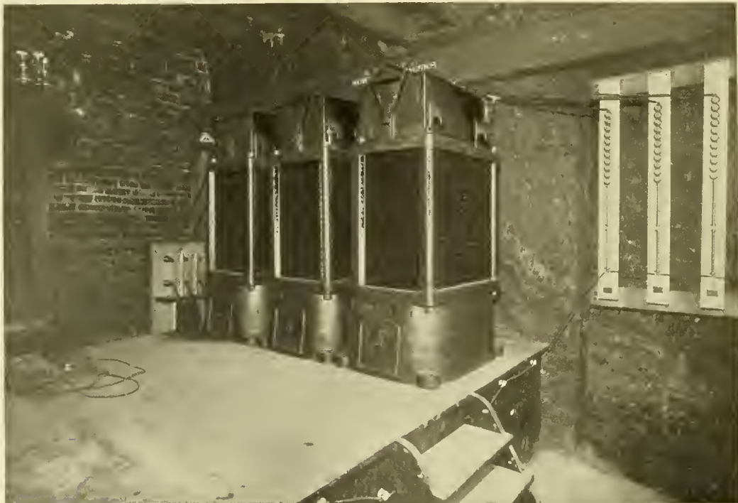
FIGURE 2—STATIC TRANSFORMERS AT BUFFALO.
