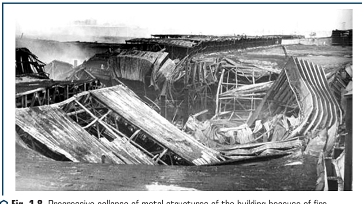
○ Fig. 1.8 Progressive collapse of metal structures of the building because of fire
