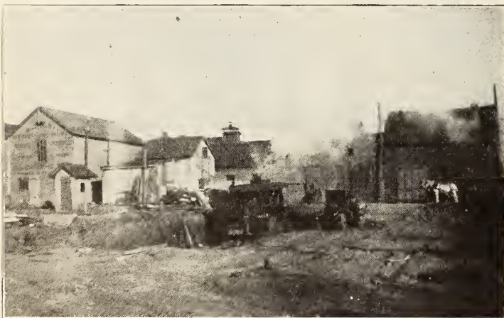
Excavating for the New Y. M. C. A. Building on the Same Lot Where the Pictures Were Shown.
