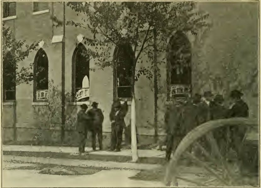
FIG. 2.— EXTERIOR OF CHURCH, SHOWING WRECKED MEMORIAL WINDOWS.
