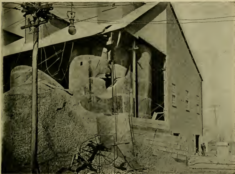
FIG. 6.— SHOWING THE DAMAGED STORAGE TANK.
