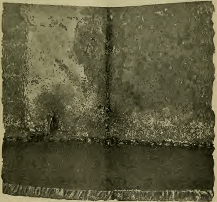
FIG. 3. WELDING OF HEAD TO SHELL. NOTE THE ROUGH CHARACTER OF THE WORK.
