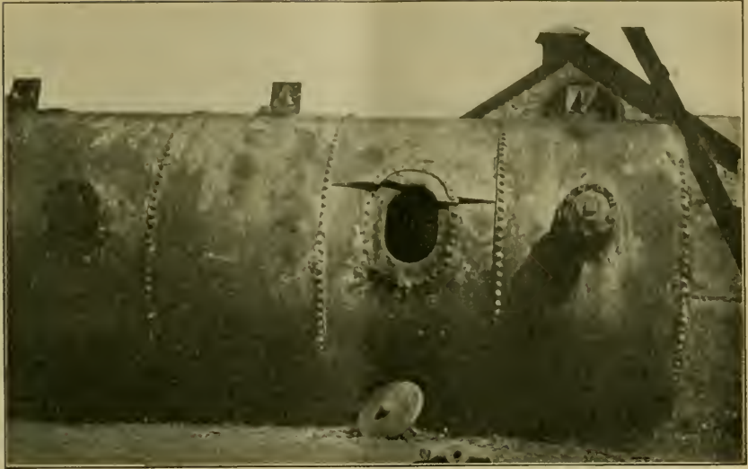
FIG. 2. SHOWING THE BROKEN MANHOLE FRAME OF BOILER 302.
