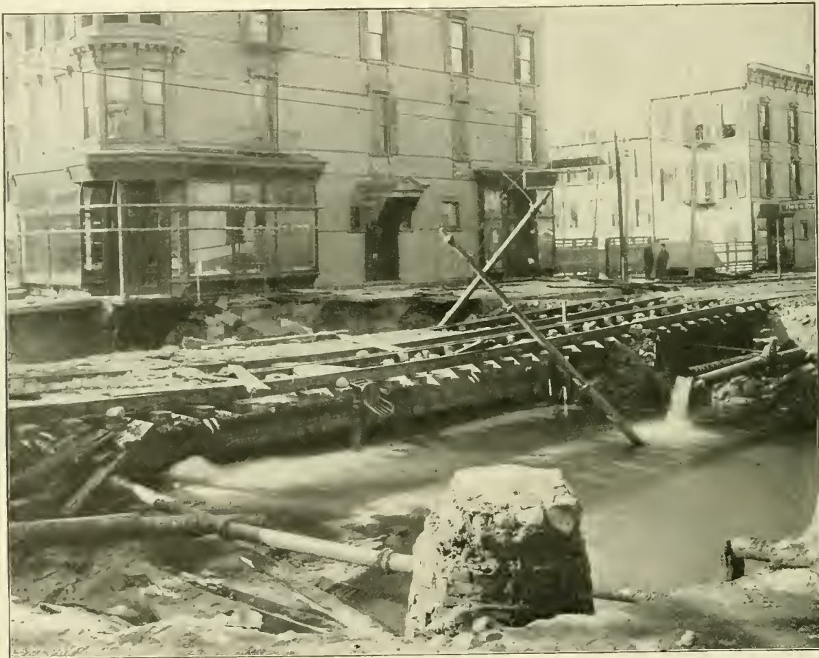
BREAK IN A 48-IN. WATER MAIN IN BROOKLYN, N. Y.
