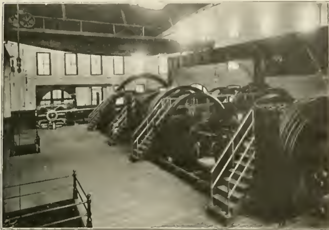
ENGINE ROOM, 12TH ST. AND BLUE ISLAND AVE.
