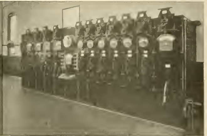
FIG. 13—SWITCHBOARD, 4½ ST. STATION.
