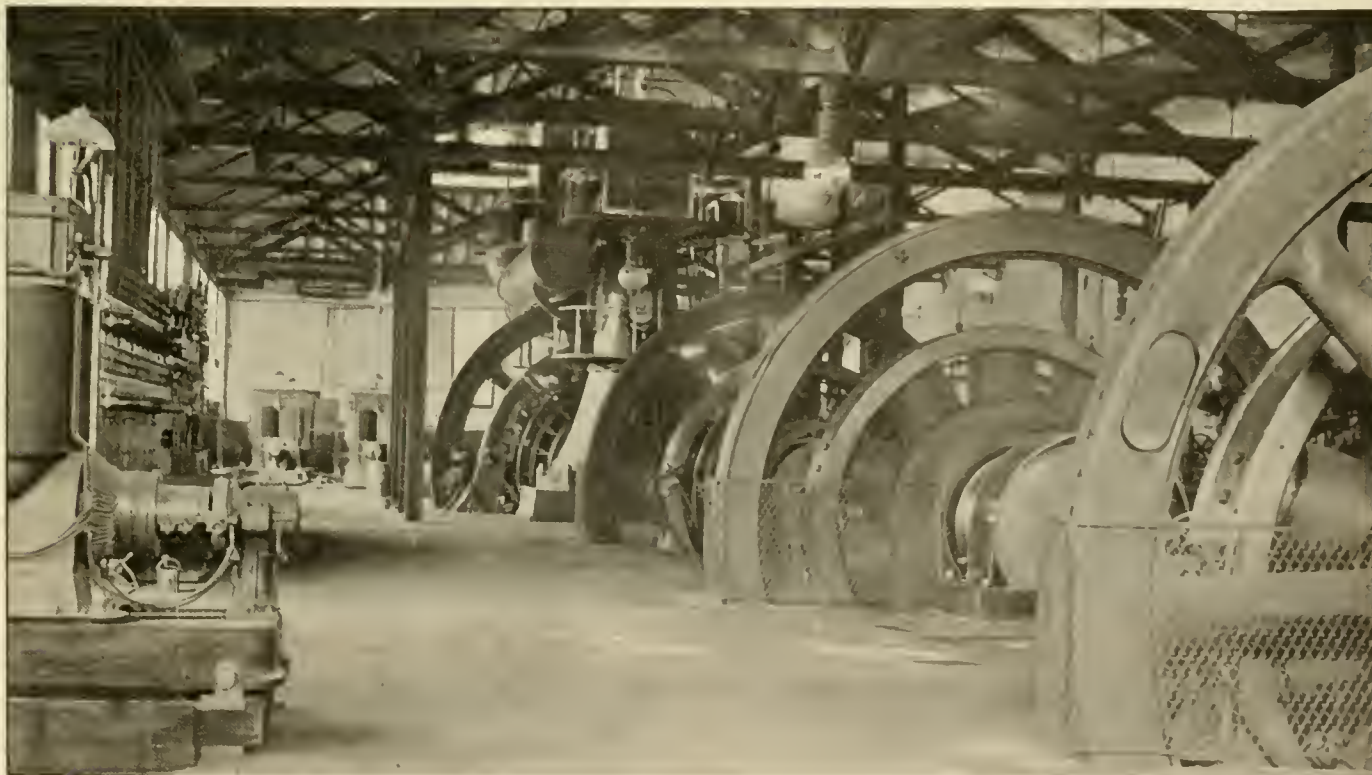
ENGINE ROOM—LOUISVILLE RAILWAY CO.
