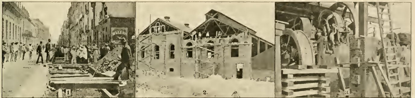
1—LAYING 60-FT. GIRDERS—TEMPORARY TRACK AT LEFT. 2—POWER HOUSE. 3—INTERIOR OF POWER HOUSE DURING ERECTION OF MACHINERY.
