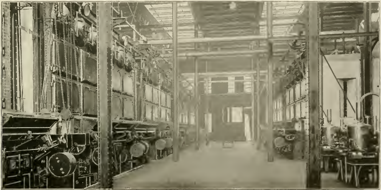
BOILER ROOM, UNION LOOP POWER HOUSE.
