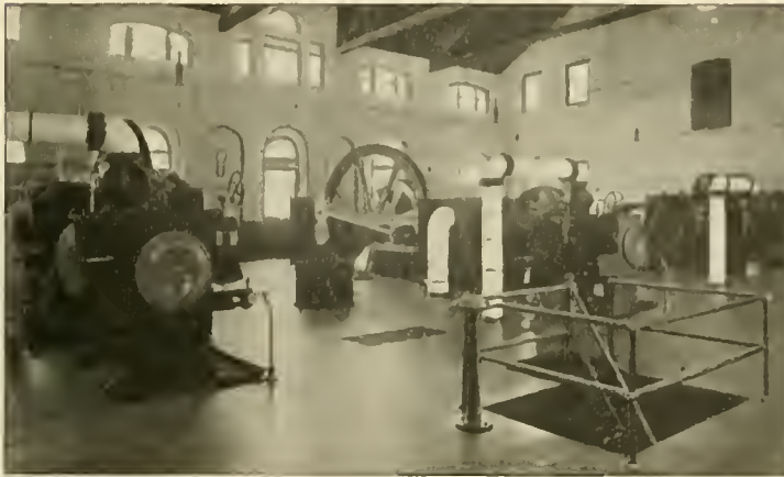
FIG. 12—ENGINE ROOM, 4½ ST. STATION.
