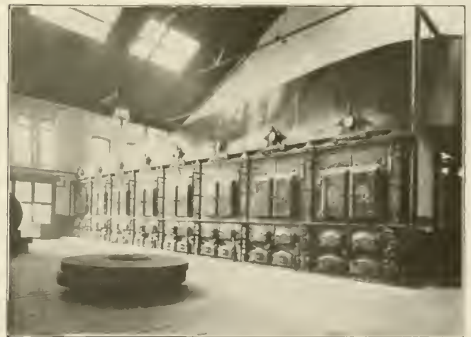
BOILER ROOM, 12TH ST. AND BLUE ISLAND AVE.
