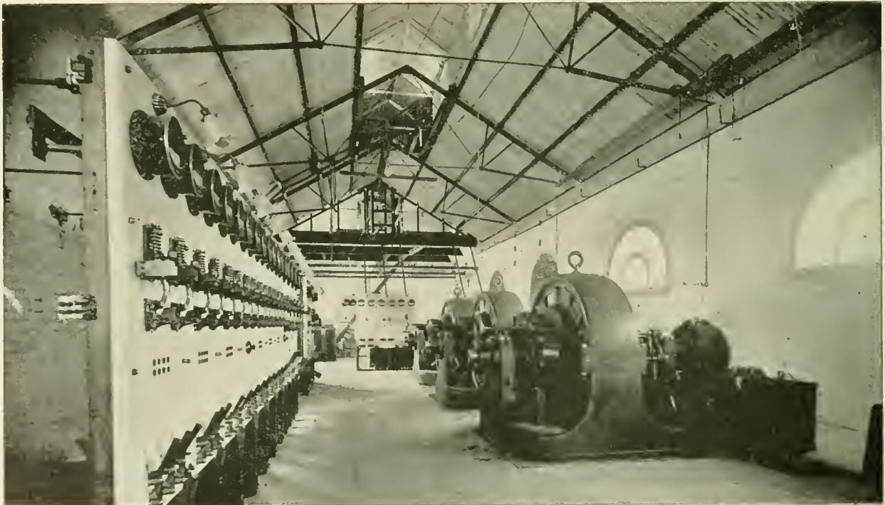
FIG. 5—INTERIOR OF LOS ANGELES SUB-STATION.
