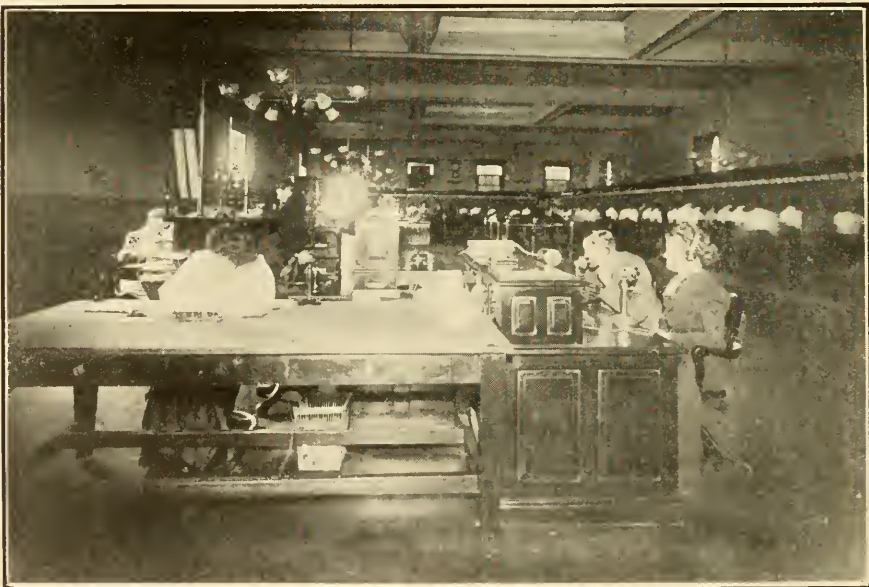
Main Office Operating Room, Showing Long Distance Chief Operator's Desk and Switchboard
