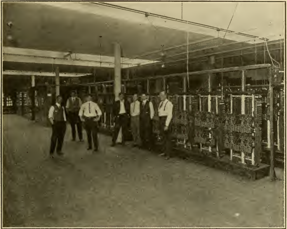
Corner of Main Switch Room, showing the few people necessary to handle thousands of Subscribers
