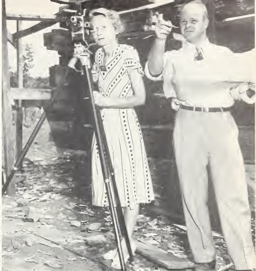
● MRS. HANSON'S interest in her husband's thesis on film is as avid as his. Construction of their log house goes on, of course, while he's at work and she carries on with the camera to insure a complete step-by-step record of its building.
