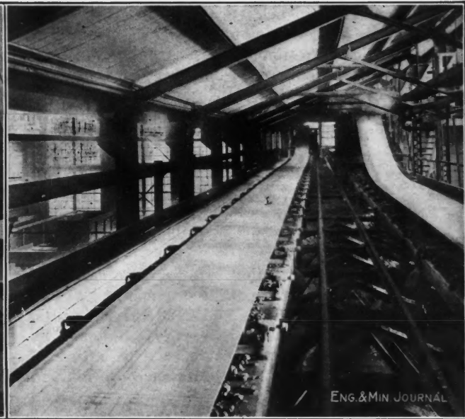
DISTRIBUTION OF CRUSHED ORE TO BINS BY 42-IN. BELTS
