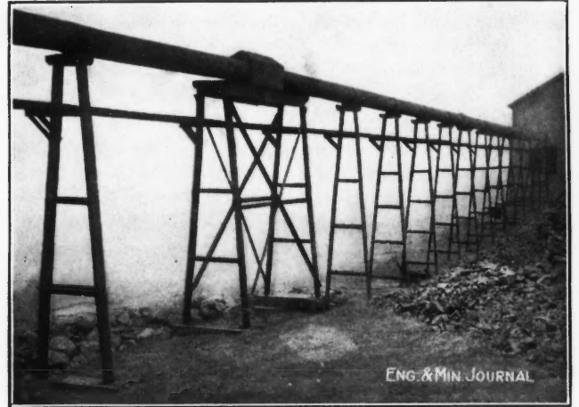
PIPE LINE FROM THE BOILER HOUSE
