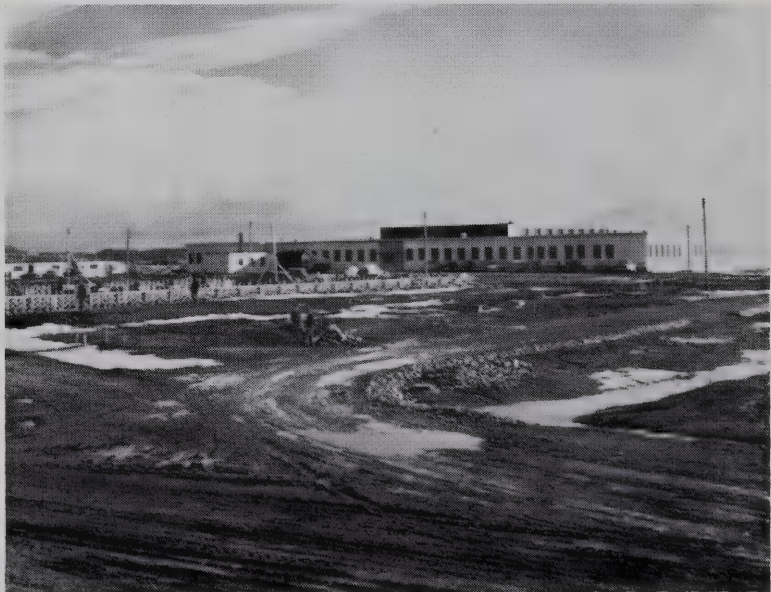
A view of the maximum security area, Calgary Provincial Gaol, at the start of construction of Phase II. The wing comprising Phase I may be seen in the background.
