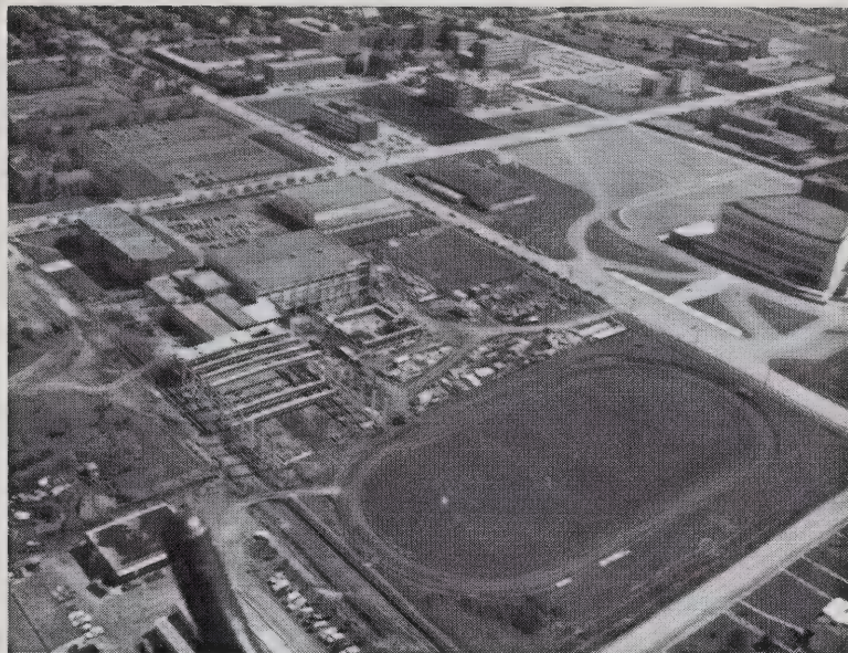
A view of the University of Alberta, showing the Physical Education Building under construction.
