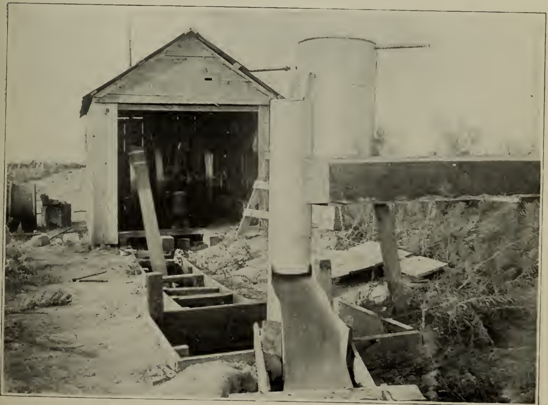
FIG. 2.—IRRIGATION PUMPING PLANT OF R. W. BRISCOE, 4 MILES EAST OF MALAGA, FRESNO COUNTY, CAL.
