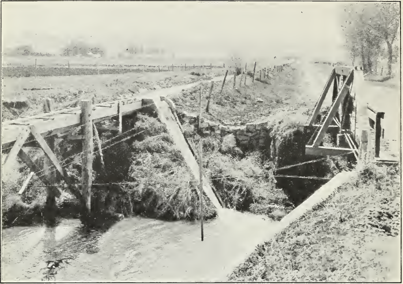
FIG. 1.—FLUME CARRYING TAIL OF LITTLE CACHE LA POUVRE DITCH OVER DRY CREEK.
