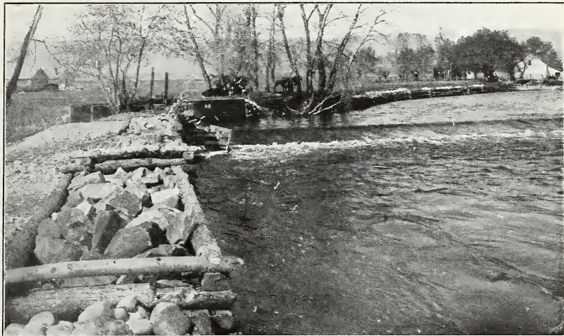
FIG. 1.—ROCK-FILLED CRIBS USED AS RIVER PROTECTION AT THE HEAD OF THE ARTHUR DITCH.
