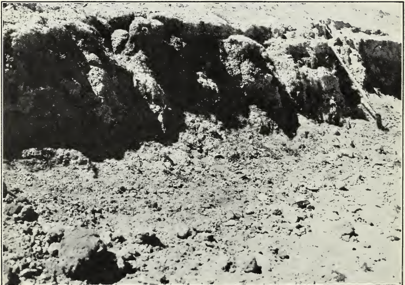
FIG. 2.—EFFECT OF WAVE ACTION ON THE INNER SLOPE OF THE DAM OF NORTH POUDE RESERVOIR No. 15.
