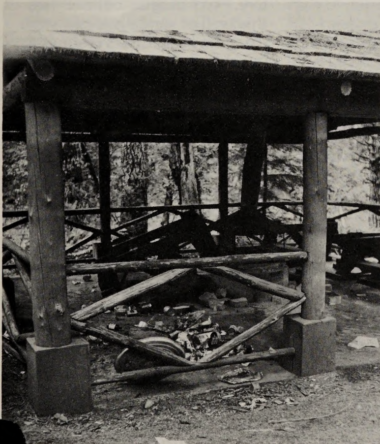
Vandalism by several teen-aged boys at a BLM recreation site.
