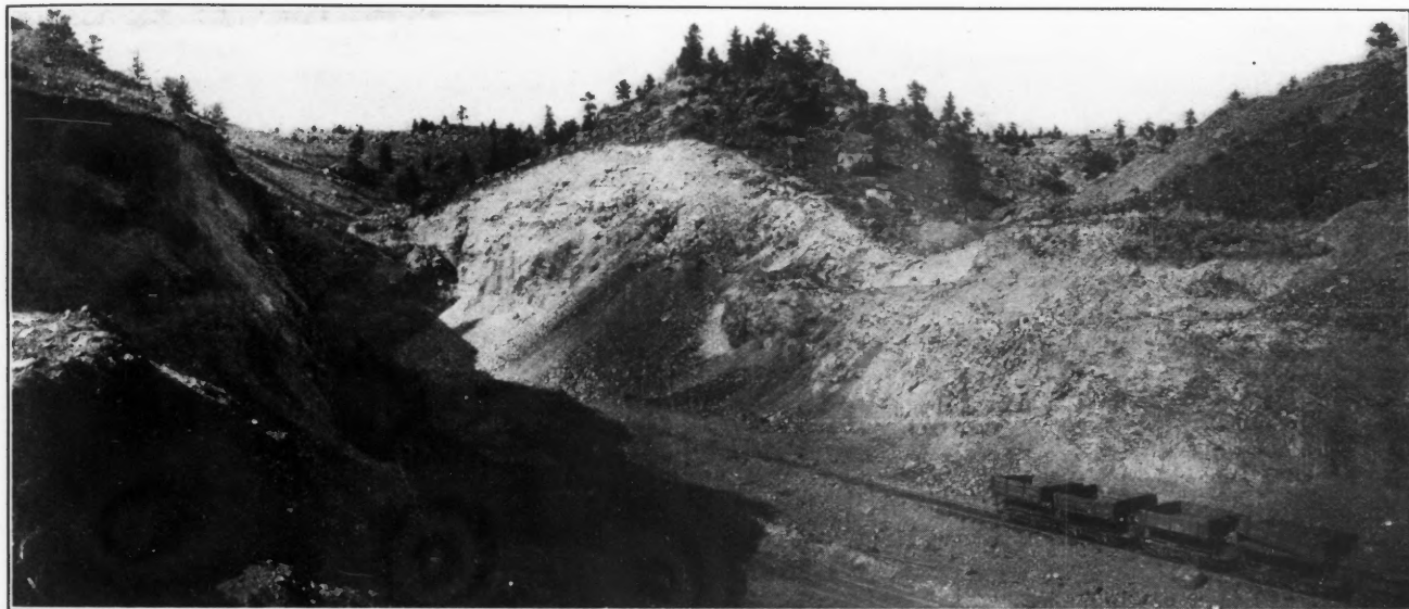
PIT NO. 2 OPERATED WITH STEAM SHOVELS. STRIPPING OPERATIONS ARE BEING CARRIED FORWARD ON BOTH SIDES OF PIT
