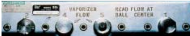
Fig. 7-29. Top of the flowmeter manifold, showing the assigned numbers imprinted for each medical gas. The numbers above the bolt holding the flow tube in place must match the number on the bottom of the flow tube. From the left, number 2 is for nitrous oxide, 4 is for low-flow oxygen-for-vaporizer, 5 is for high-flow oxygen-for-vaporizer, and 1 is for metabolic oxygen. Switching flow tubes can be disastrous because the output of the flowmeter is determined by the specific viscosity and density of the medical gas flowing through the flow tube.
