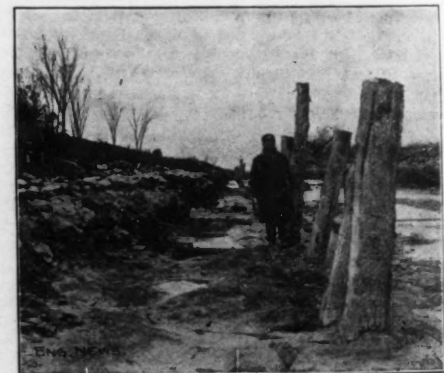
Fig. 4.—View Showing Manner in which Piles Rose and Tipped After Driving, Jordan Level Marl Beds.
