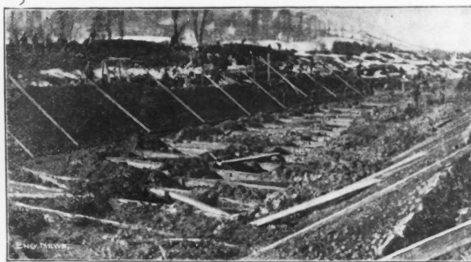
FIG. 6.—VIEW OF CANAL PRISM, SHOWING BOTTOM BRACES IN PLACE AND SLOPE WALLS UNDER CONSTRUCTION.
