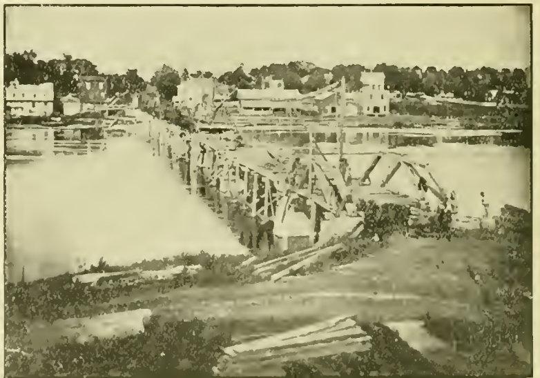
Old Photo loaned by W. E. Sparrow. CONSTRUCTION OF THE NEW BRIDGE.
