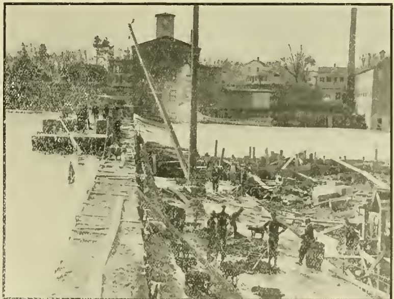
Old Photo loaned by W. E. Sparrow. CONSTRICTION OF THE NEW DAM.
