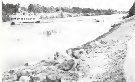
A concrete structure at the toe of the streambank, at right in photo, and a new planting protected with netting at the top of the bank protect this St. Lucie Canal streambank from erosion.
