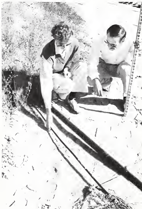
Helen Bowdoin, an SCS volunteer, and Ray Hisaw, an SCS soil conservation technician at the Tulsa, Okla., field office, look where gully erosion has exposed underground utility lines.
