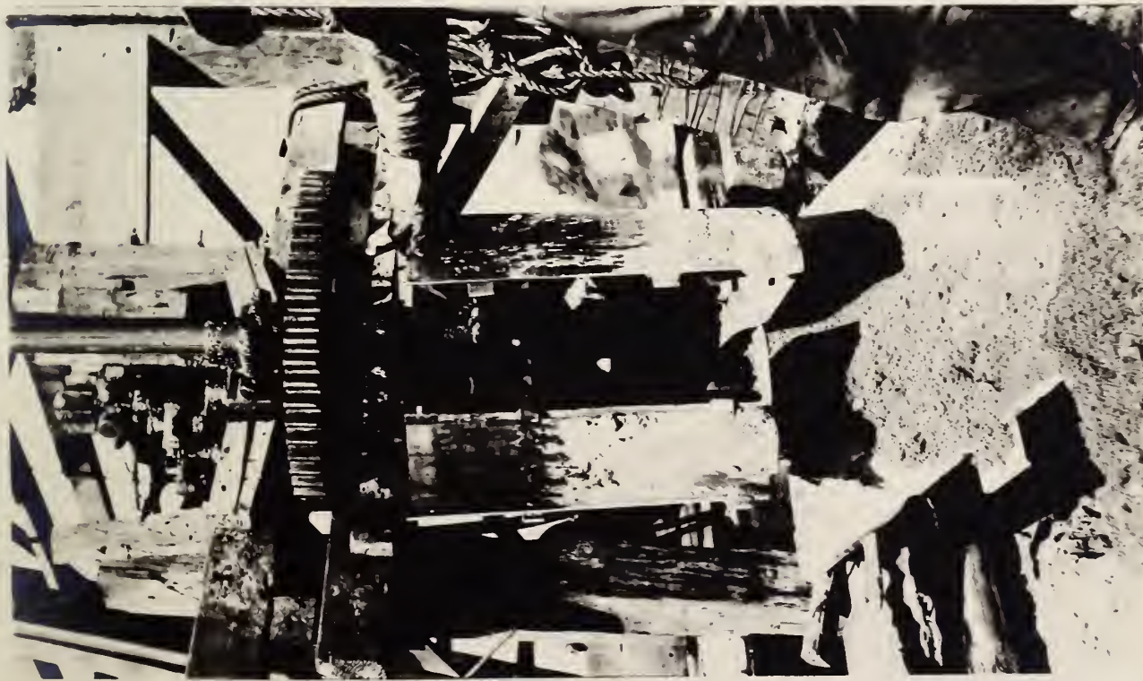
FIG. 1A - THE CYLINDRICAL BUCKET OF THE AUGER WAS PROVIDED WITH A HINGED DOOR WHICH FACILITATED REMOVAL OF THE SAND-SLAG MIXTURE.
