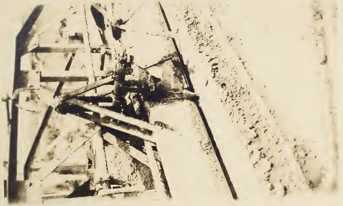
FIG. 2B - THE V-PROJECTION ON THE TAMPING BOARD OF THE LAKEWOOD MACHINE FORCES THE LARGE ROCKS AWAY FROM THE GROOVE SO AS NOT TO INTERFERE WITH THE CENTER-LINE GROOVING TOOL SHOWN IN FIG. 2A.
