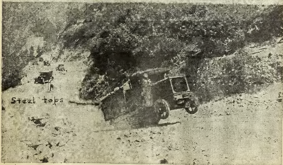
Figure 1. - (Top) General view of the topography of the project. (Center) Gas-air shovel loading the steel-bodied Linn tractors from a hard strata of granite. (Bottom) Linn tractor, with wood body extended by steel tops, tipping up on a 30 per cent grade.
