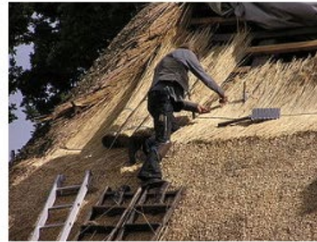
A German roofer installing a reed roof (he is wearing the tradition
