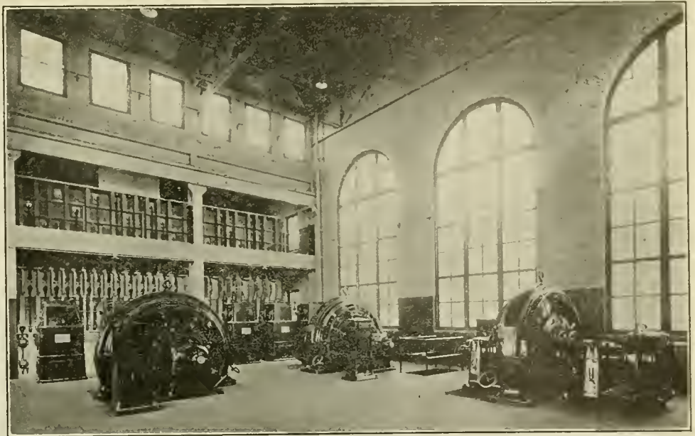
INTERIOR VIEW OF TYPICAL SUB-STATION—L. I. R. R.
