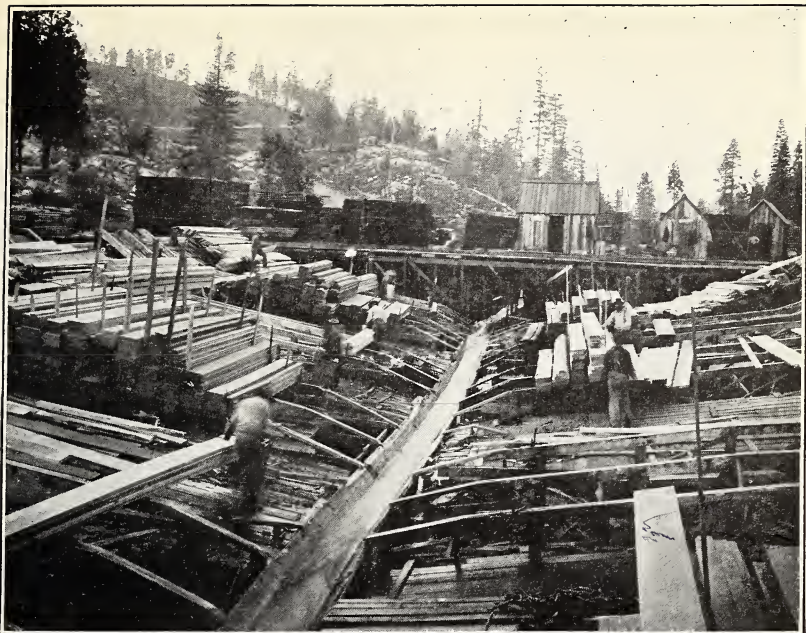
FIG. 1.—BRAILING AND ACCOURTRING LUMBER AT THE UPPER END OF A FLUME. Note the sloping "ways" on which the brails are slid into the flume after being clamped.
