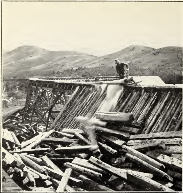
FIG. 1.—A "SNUB" IN OPERATION, THROWING CROSSTIES OUT OF FLUME AT RAILROAD LANDING BY PRESSURE OF WATER. Man present to prevent material jamming.
