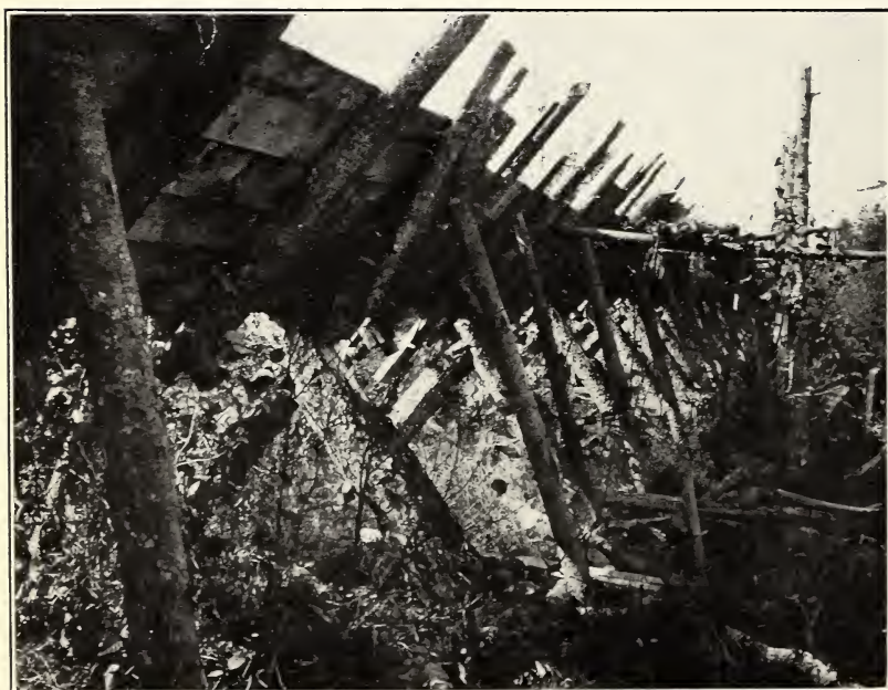
FIG. 2.—CRUDE FORM OF FLUME CONSTRUCTION WHERE ONLY THE LINING IS OF SAWED LUMBER, THE REMAINDER BEING CONSTRUCTED OF SMALL ROUND TIMBER AND POLES.
