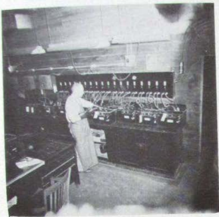
BATTERIES NEED CHARGING
