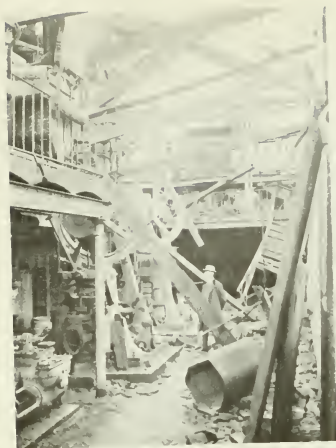
Fig. 4. Wreckage at a sugar refinery in Chauny.
