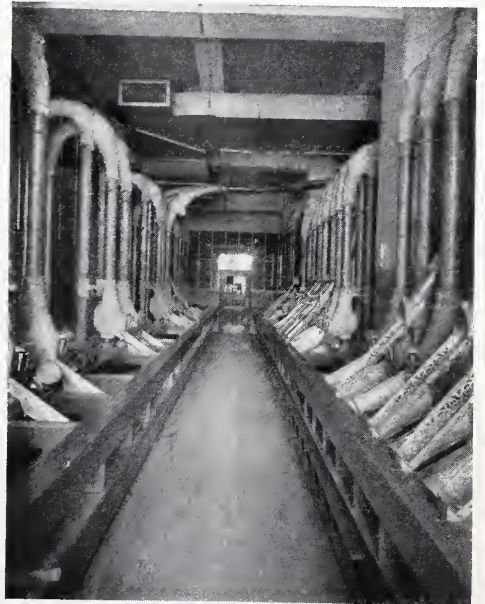
STORE SERVICE TUBE ROOM.
