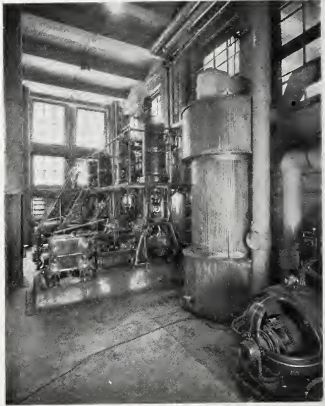
Pump Room—Ice Machine. THE CURTIS BUILDING.
