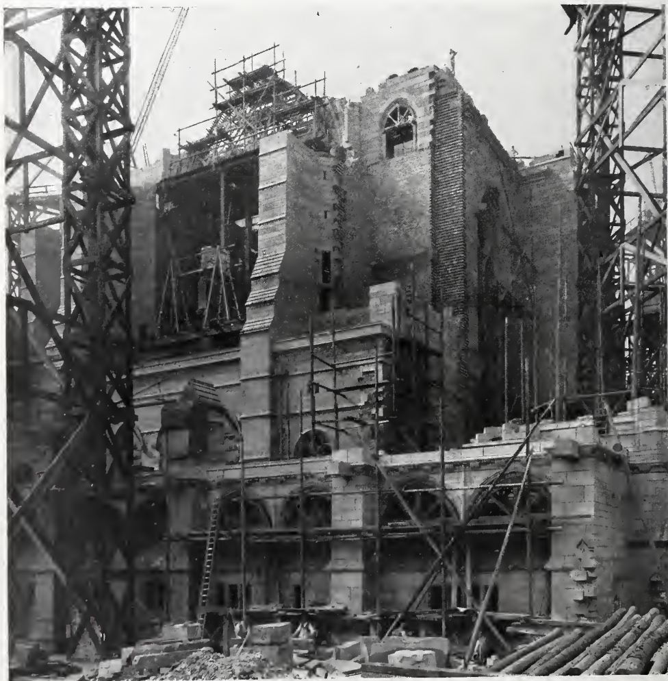
By permission of Messrs. Morrison & Son. EASTERN ELEVATION—SHOWING LOWER PART OF CHAPTER HOUSE ON THE RIGHT—LIVERPOOL CATHEDRAL. G. G. SCOTT, ARCHITECT.
