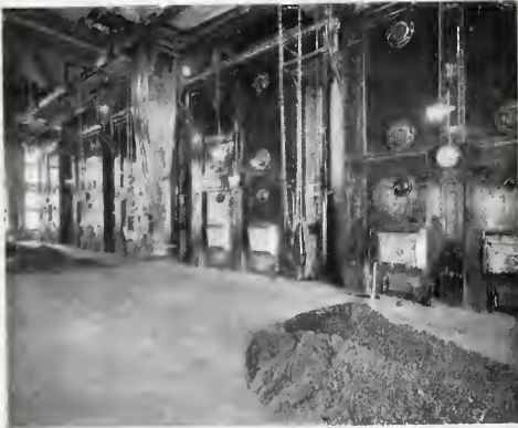
THE BOILER ROOM.
