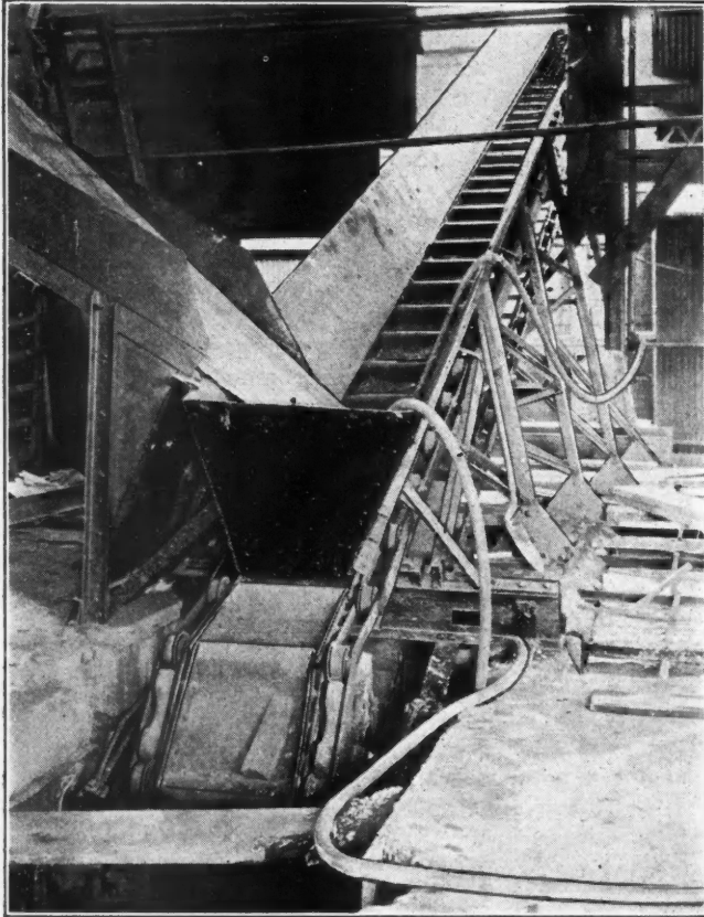
PAN CONVEYOR FOR CARRYING SINTER TO BINS
