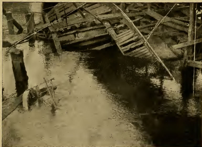
Another bridge at Termonde destroyed by shell-fire.
