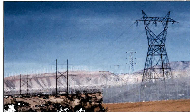
Photo 13. Segment 6 by Devers Substation
