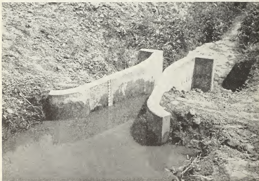
FIGURE 22.—The 9-inch flume in action, free flow, with a discharge of 3.40 second-feet. This structure is shown in figures 19 and 20.
