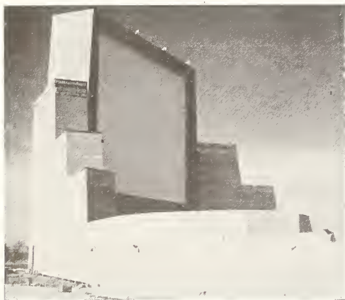
The Springfield drive-in screen is mounted on a sturdy structure of laminated lumber. It is 75 feet high.
