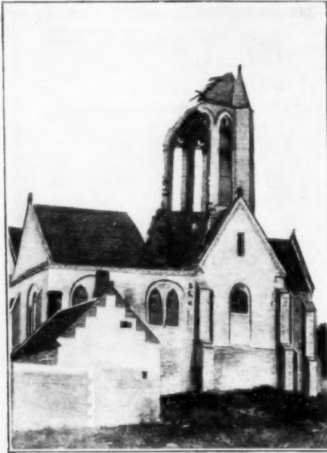
The Structure After the Dynamiting of the Belfry the greater part of the heavy stone and debris toppled inward. The operation was considered very successful.
