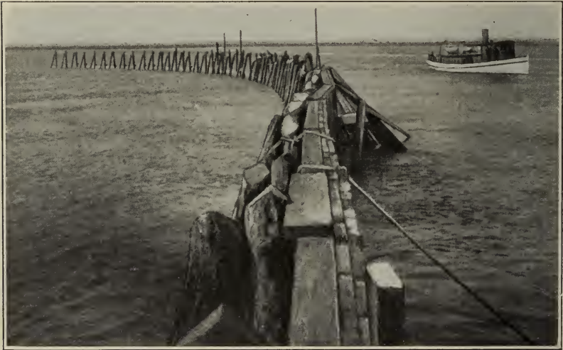
Fig. 2. Western half of the same jetty, showing planking undermined by the deep scour, 1901.
