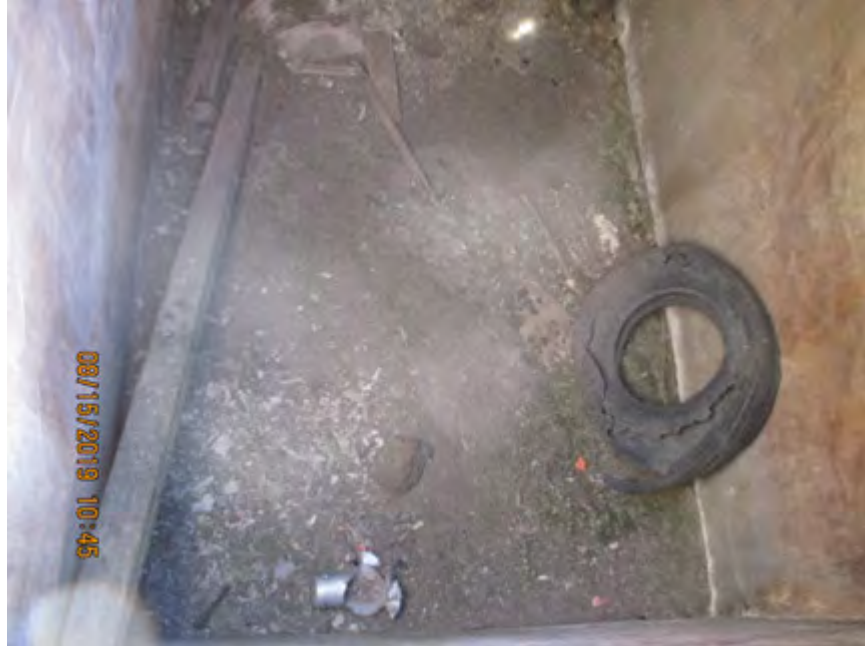
Photo 40. Solid waste and tire inside concrete basin. Photograph taken by Bryce Anderson on 8/15/2019.
