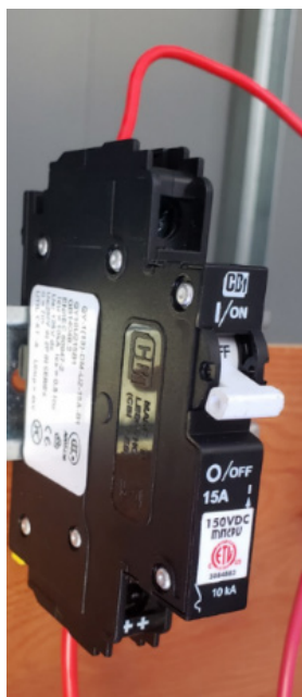
Figure 27. Switch to allow self-powering of the fuel cell
