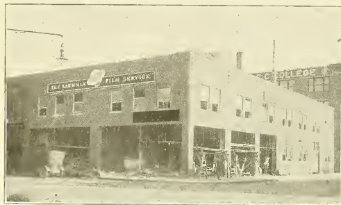
The Laemmle Service Company's new building in Des Moines, Iowa, as it now appears under construction.
